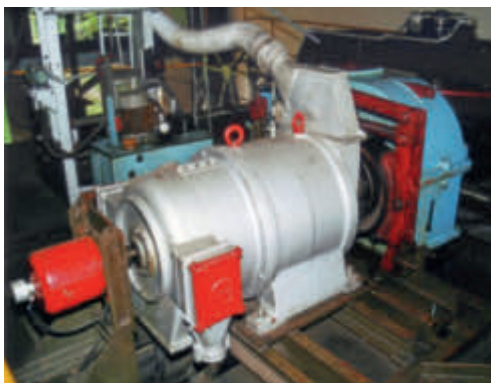
The 62.5 kW overhead drive with the service brake and the gearbox (blue) in the bottom station
