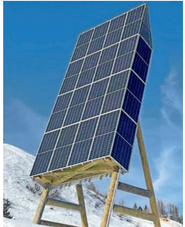
The tower-shaped PV-Pappel , the PV installation located on the Gerlitzten in Carinthia at 1,770 m above sea level
