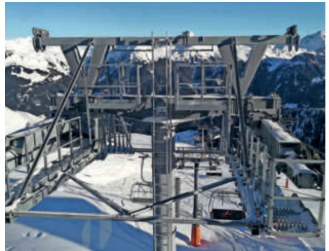
Example of a tower head with platforms for safe working on the sheave trains
