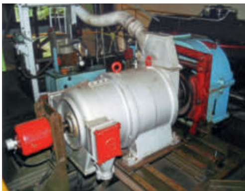
The 62.5 kW overhead drive with the service brake and the gearbox (blue) in the bottom station
