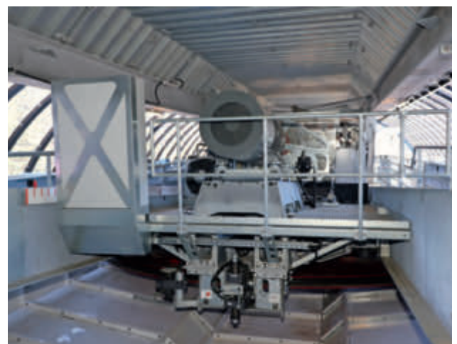
Hydraulic tensioning for the overhead drive unit in the bottom station
