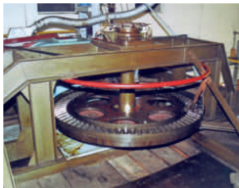
Power transmission from the gearbox to the bullwheel is via an open gearwheel and ring gear.
