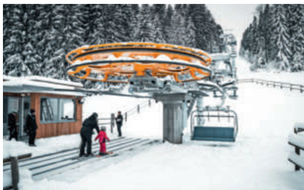
Bottom station with loading conveyor for the new CF4 Ruška fixed-grip 4-seater chairlift in Mariborsko Pohorje (SLO)
