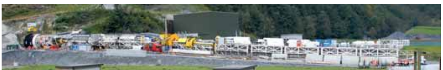
Rotary boring machine for driving the tunnel for the supply funicular serving the Limmern power plant
